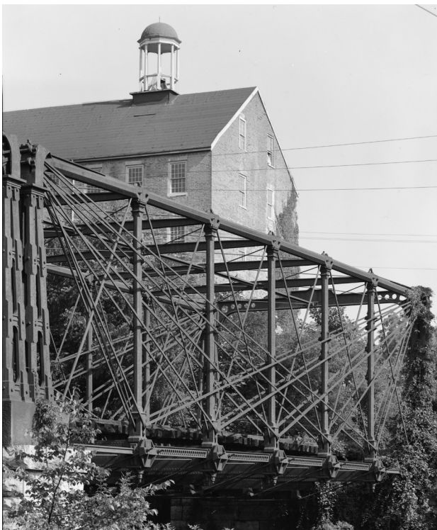
7. General view of truss on east side of bridge, Baltimore & Ohio Railroad, Savage, Howard County. Fotografía de William E. Barrett, 1970. Library of Congress, Prints & Photographs Division, HAER MD,14-SAV,1-6
